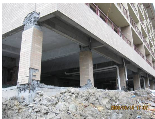
(b) 底层柱铰 (b) Column plastic hinges at the first story
