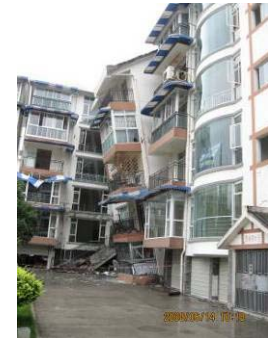
Weak story collapse of a RC frame
