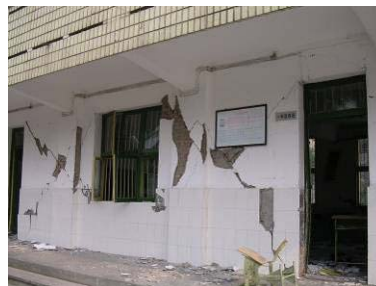
Severe damage in the load-bearing walls and columns of the teaching building of Huayuan St. Middle School, Jiangyou
