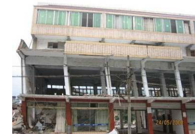
Plastic hinges in frame columns, Nanba
