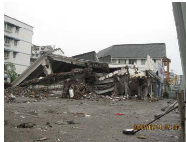
Collapse of a RC frame with a heavy roof, Dujiangyan
