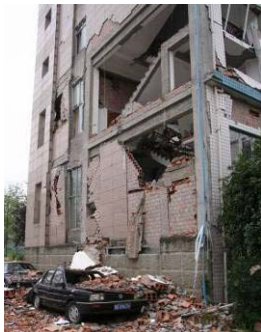
Filler wall collapsed, Dujiangyan
