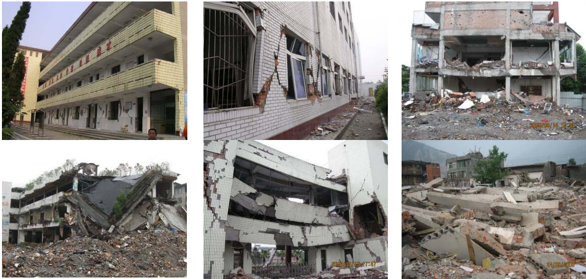
Fig 12 Different states of building damages beyond the design point against severe earthquake
